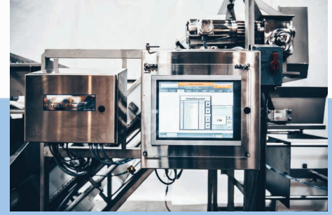
B&R® Automation Control
